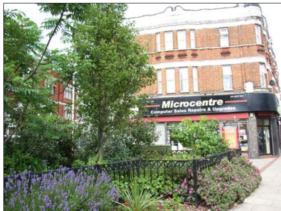
Parapet painted to conceal brick defects
