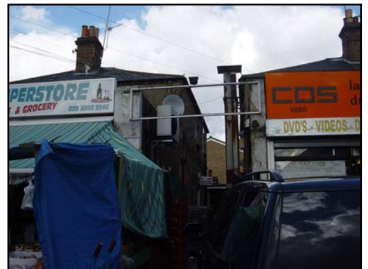
Retail units in Frogmore Green are disfigured by incompatible shopfronts and signage
