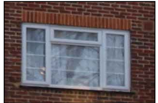
Inappropriate window replacement
