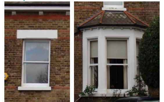
Sash window with stuccoed lintel and stuccoed canted bay in Mount Avenue
