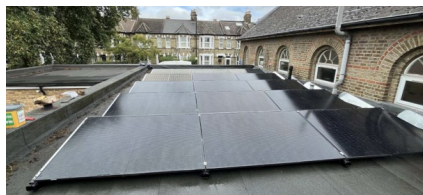
Several groups have used grant funding to help install solar panels. Above: at the William Hobbayne Centre in Hanwell.
