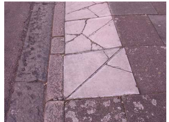
Granite kerbs with broken paving
