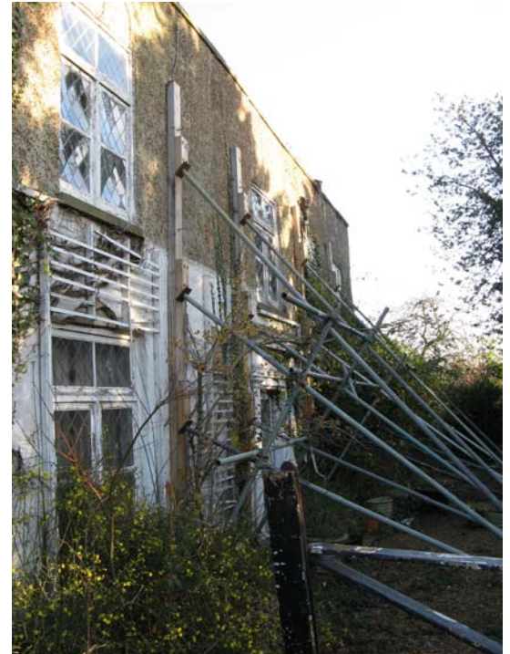
No 134 Church Road – a listed 'Building-at-Risk' requiring urgent attention
