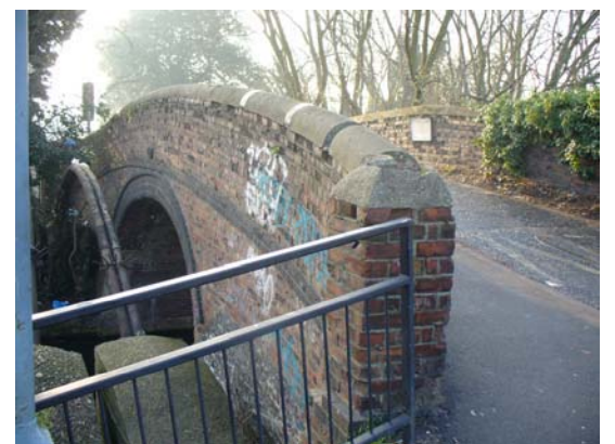
The narrowness of the carriageway over Old Oak Bridge may create pressure for replacement
