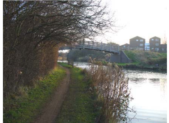
Canal towpath is in poor condition in some areas
