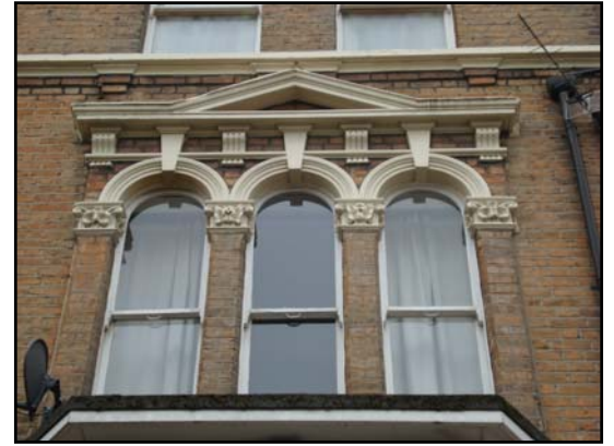
Italianate, tripartite window with stuccoed pediment and arches with key stone supported by decorative capitals
