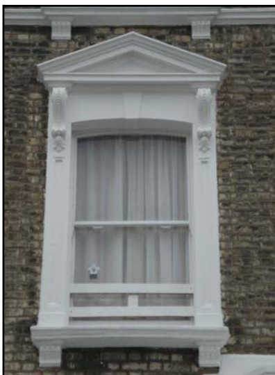
Mid-Victorian, Italianate window with stucco pediment, key stone, corbels and projecting cill
