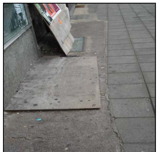
Poorly treated and maintained shop forecourts
