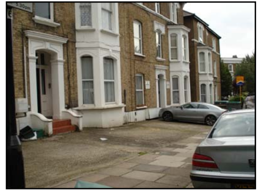
Conversion of the front yard to hard standing and loss of boundary treatment
