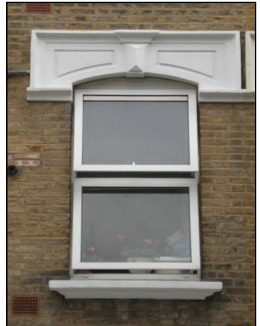
Inappropriate window replacement with UPVC
