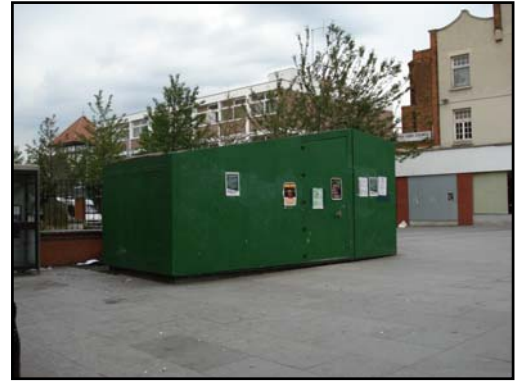
Large service cabinet in the proximity of St Mary's Church graveyard spoiling the setting of the listed building
