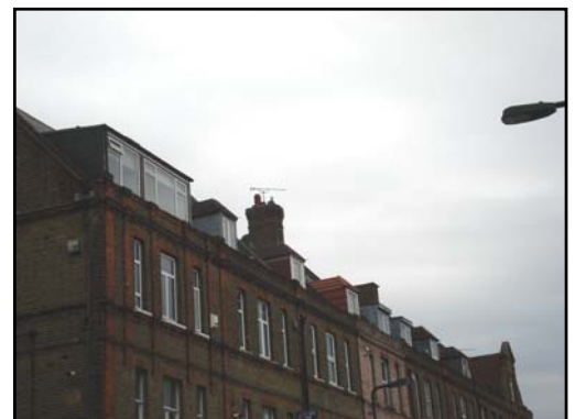
Parade of uncoordinated front-dormer windows disrupting the roofline
