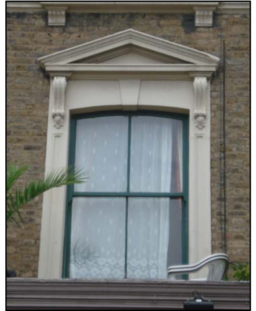
Typical mid-Victorian sash (2/2) with classical stucco trimming with central key stone, side corbels and top pediment
