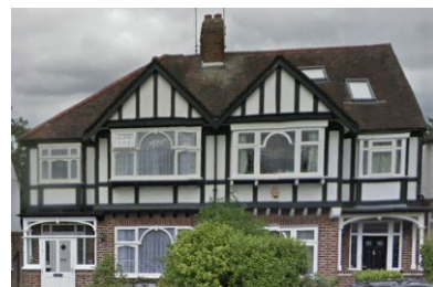
Changing from hipped to gabled roofs can unbalance appearance in the streetscape.
