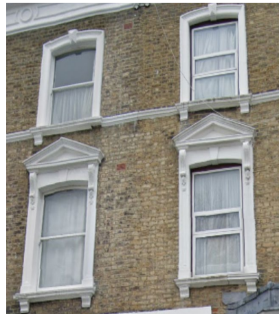
The original timber sliding sash windows to the left have been replaced with inappropriate PVC-U windows to the right.
